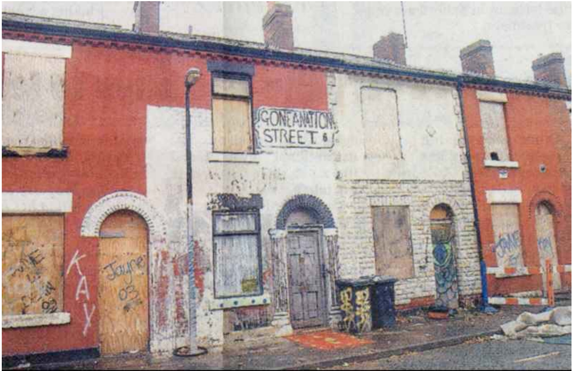
Current state of Langworthy homes – quality brickwork and construction, badly neglected
